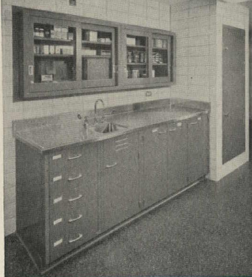
Sub utility room
