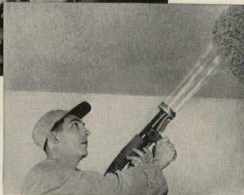
Applied in one operation, SPRAYED "LIMPET" ASBESTOS combines in mid-air with water from special spray gun.
