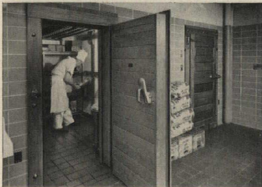
Both walk-in refrigerators are insulated with Styrofoam.
