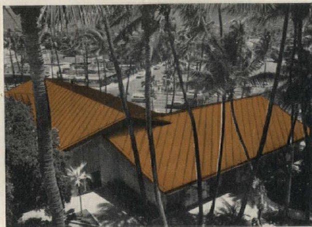
MOST UNUSUAL ROOF EFFECT is obtained by running batten seams on the diagonal. Copper was furnished by Revere Copper and Brass Incorporated. Architect: VLADIMIR OSSIPOFF, F.A.I.A.
