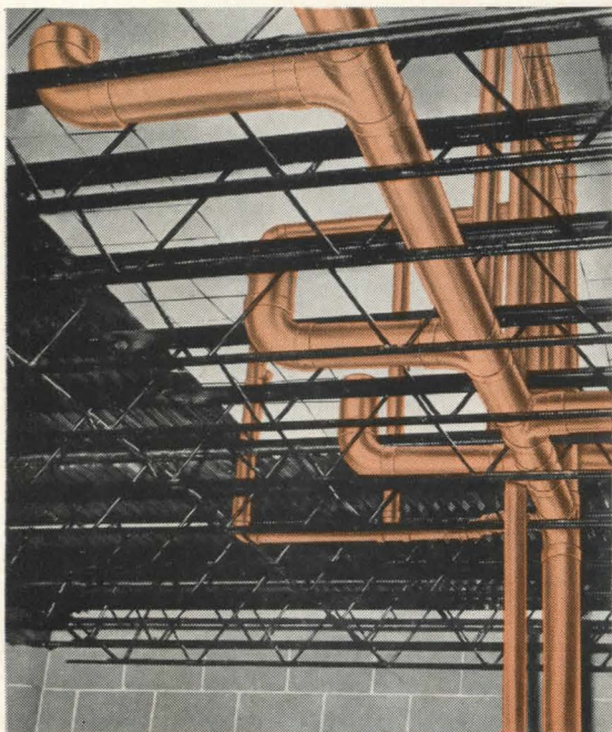
COPPER SANITARY DRAINAGE LINES roughed-in among structural members at Gower School. This space-saving installation would have been impracticable with heavy, bulky pipe requiring threaded or caulked joints.
