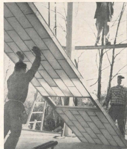
Four-man team from Boss Glass Company, Caldwell, N. J. enclosed 1000 sq. ft. of wall area a day. Men had never installed Kalwall before. 14' x 4' panel unit is so light one man can push it upright. Panels are held in place by channels bolted to floor and roof.
