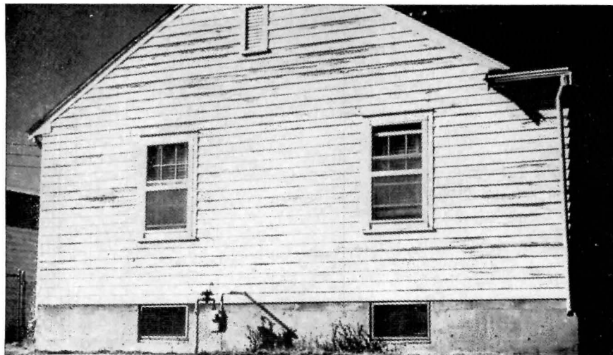
Blistering and peeling paint is one of the most common types of damage caused by the collection of excessive vapor in the side walls.
