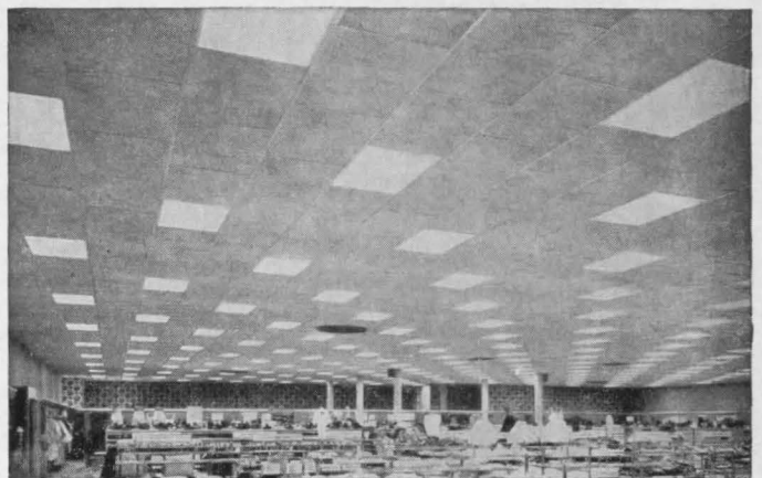
Smithcraft 2'-wide Metro Troffers provide 75 footcandles of extremely even illumination throughout Beerman's Department Store, Dayton, Ohio. Metro Troffers are lay-in troffers for inverted "T" Grid ceiling systems.
