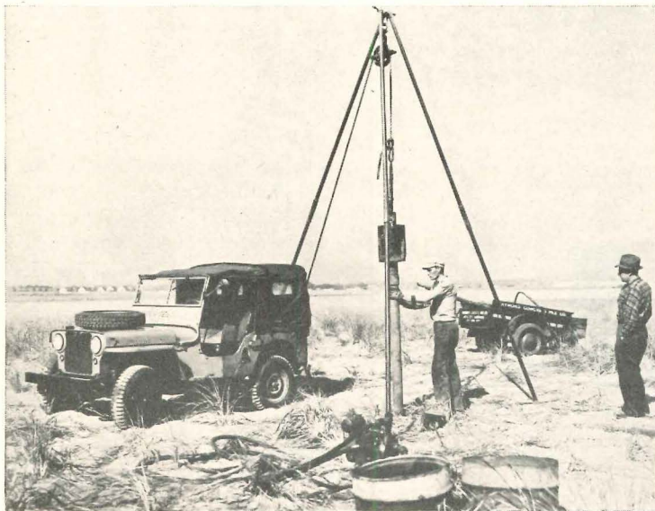
Soil investigations for heavy structures call for more complicated equipment than the auger. Casing is being driven into the ground by the "standard boring" method prior to taking a sample. The steps are outlined above
