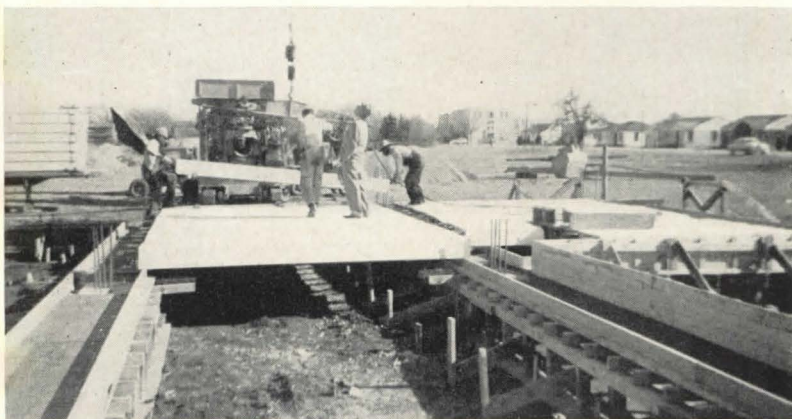
Above: Crane not shown in photo lifts joists from load at left and lowers them into position, spanning between beam formwork. Below: Second floor joists near one of the columns
