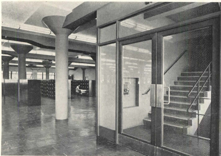
Interiors are simply and boldly done. Ducts and columns are frankly exposed and gaily painted. Columns are dark green, walls a lighter green, air conditioning ducts red
