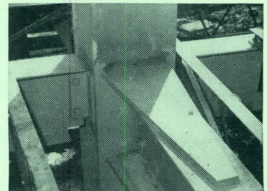
Fig. 2. Simpler Detail Speeds Erection. Clip angle is shop welded to column for bolting beam in the field. Outside cover plates are then field welded to top and bottom flanges and the top plate to column in flat position with Lincoln "Fleetweld 5" electrodes. Bottom plate is shop welded.
