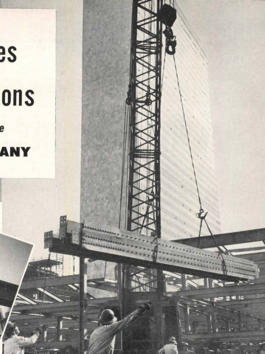
AGAINST A BACKGROUND of the completed UN Secretariat Building, for which American Bridge Company fabricated and erected 13,800 tons of structural steelwork, two bridgemen direct the unloading of steel columns and beams for the North Parking Space at the UN site.
