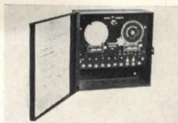
Typical centralized program panel.
