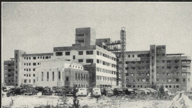
Mercy Hospital, Miami, Florida. Commencing of THOROSEAL applications. Architect—Steward and Skinner, Miami, Florida. Contractor—J. Y. Gooch Co., Miami, Florida.
