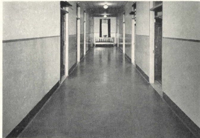
3. A corridor in the same hospital showing an installation of battleship linoleum now in use over thirty years! Proved long life where traffic is heavy . . . always clean and sanitary.
