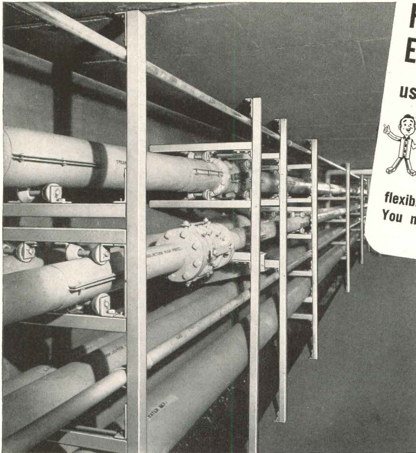
Unistrut steel channel and fittings, roller pipe supports and concrete inserts at work in a tunnel installation at G. D. Searle & Co., Skokie, Illinois, manufacturers of ethical pharmaceuticals.
