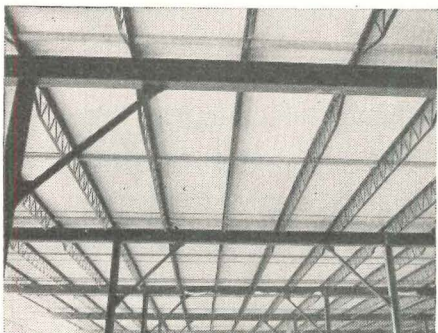
Light steel framing for 53,760 sq. ft. of Cemesto for Watson Terminal Warehouse Company, Youngstown, Ohio.
