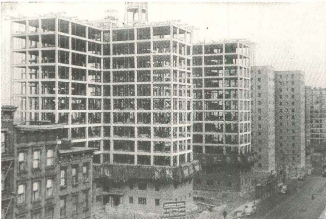
LOW COST —The Gold Bond Solid Partition System, approved by New York City's Housing Authority, helped the successful bidder figure his costs down to a minimum. These are the Amsterdam Houses in New York—1084 apartments.
