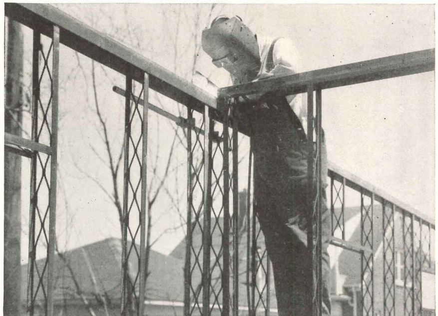
Fig. 1. Arc welding steel panels to form the side walls. Panels are made from 4" Bethlehem expanded steel studs.
