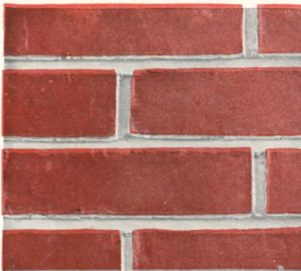
A weathered joint does not always pack the mortar against the top brick thoroughly.
