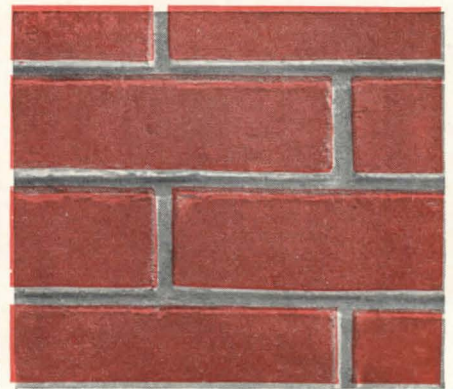
A raked joint leaves a bad shelf and often contains too little mortar especially in the head joint.
