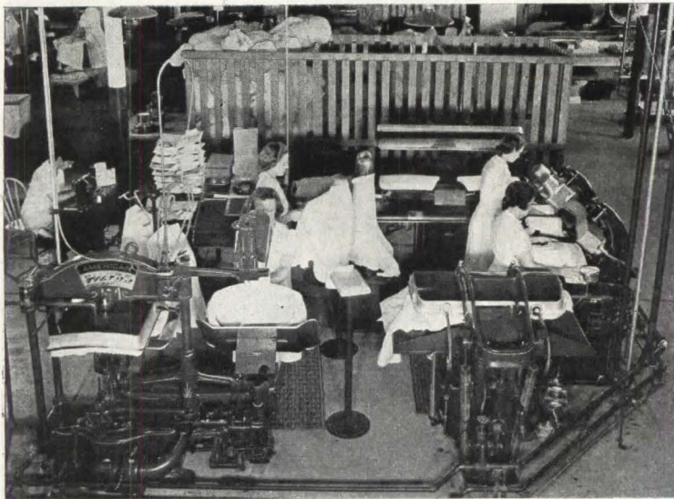
Above: The wearing apparel and finishing unit. At Left: The shirt pressing unit arranged for maximum convenience and production—note also the piping system for the various type presses
