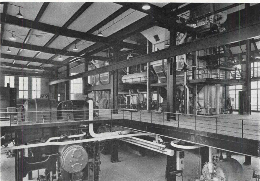
Interior of the Burroughs power plant. It was one of the first plants to break away from the common practice of putting a partition between boiler and generator rooms. Coal dust is not allowed to escape
