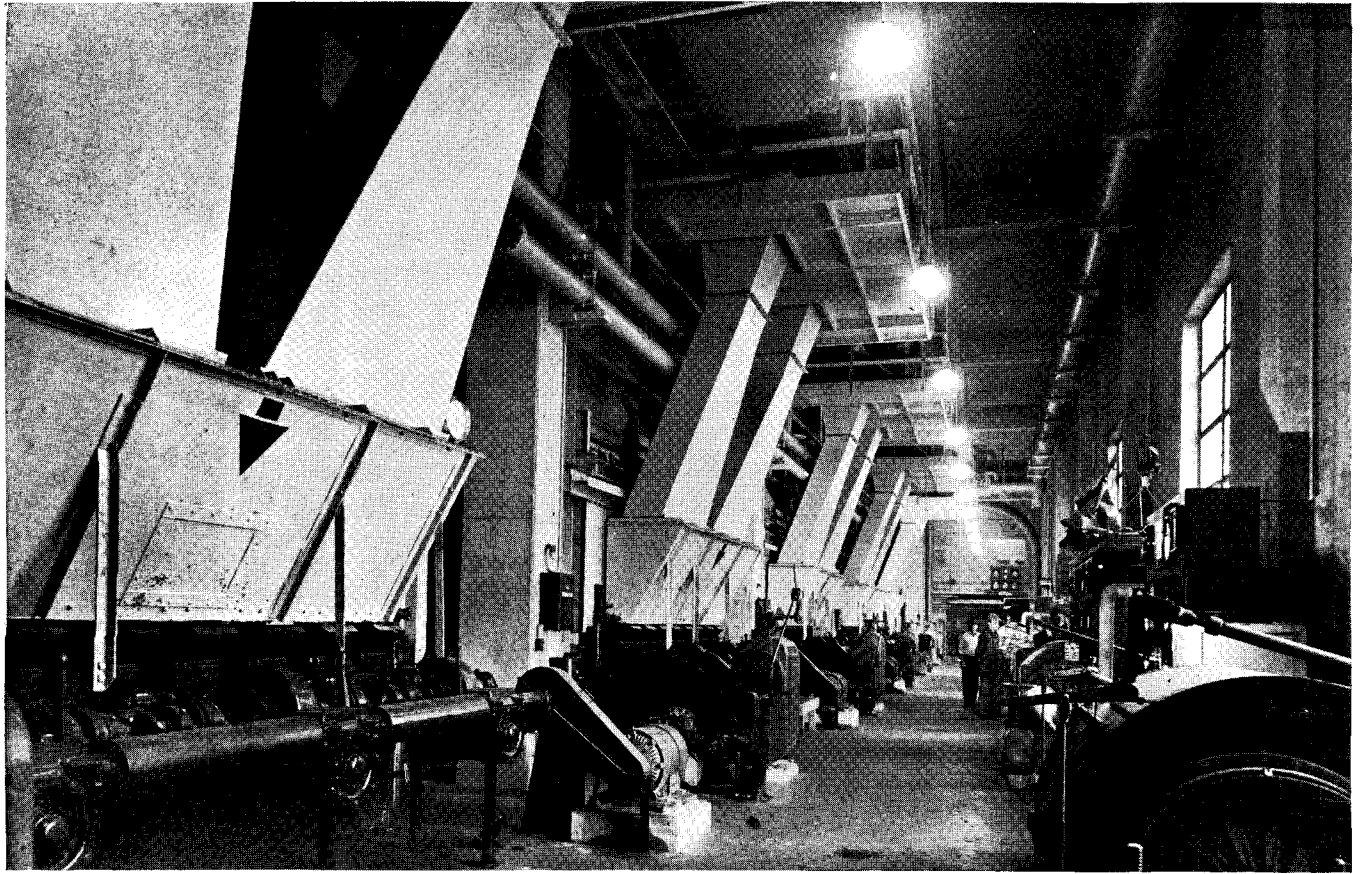
View of boiler room in separate building. Boilers are for heating only, as electric power is provided by the local utility company
