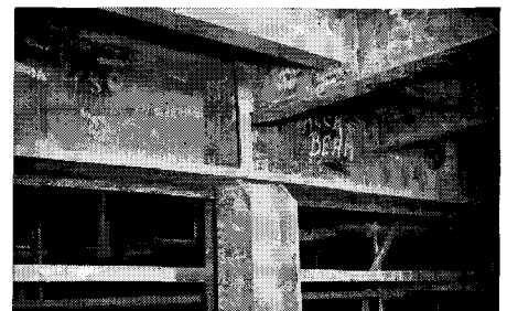
Hatch end beam supported by main pillar carries longitudinal stringers and girders, which in turn support deck beams.
