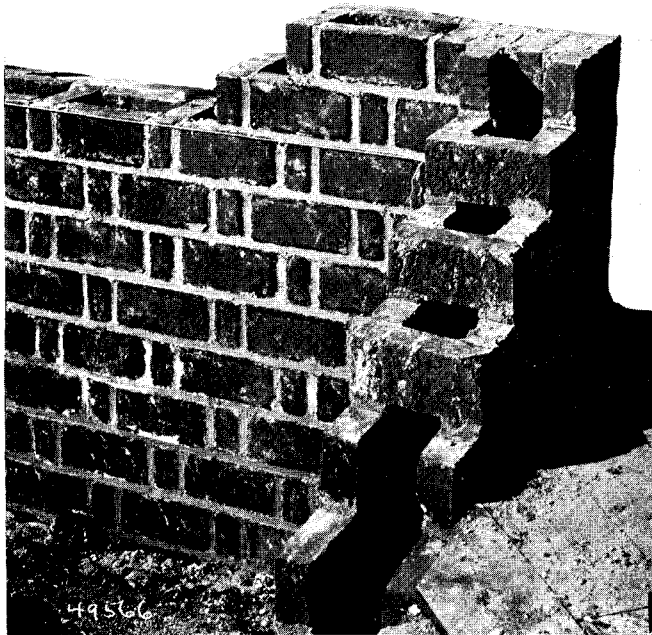
Fig. 4. Simplest of all advances in ordinary brick masonry is this hollow wall construction. Although boasting some advantages, moisture can still penetrate via headers.
