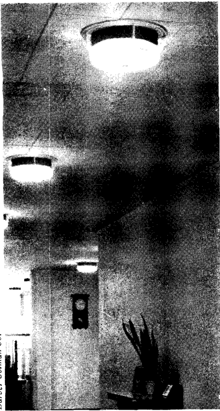
1. A combination of direct lighting with outlet for supply duct; heat generated by lighting is modified at the source.
