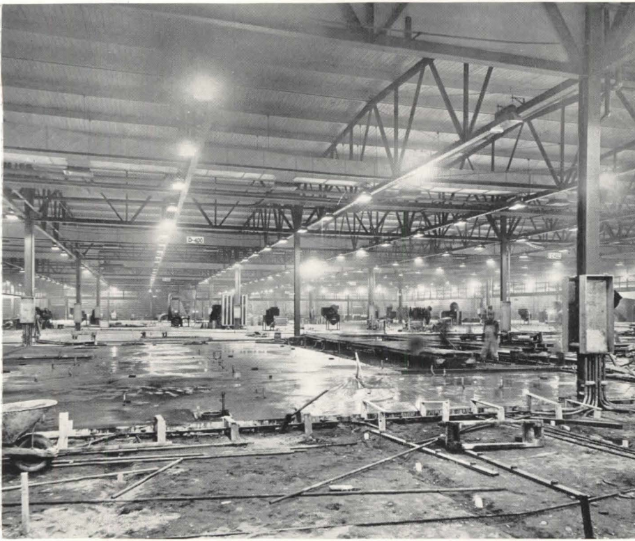
Under-floor installation of utility ducts and pipes allows greater flexibility in the economical layout of machinery and material-handling equipment.
