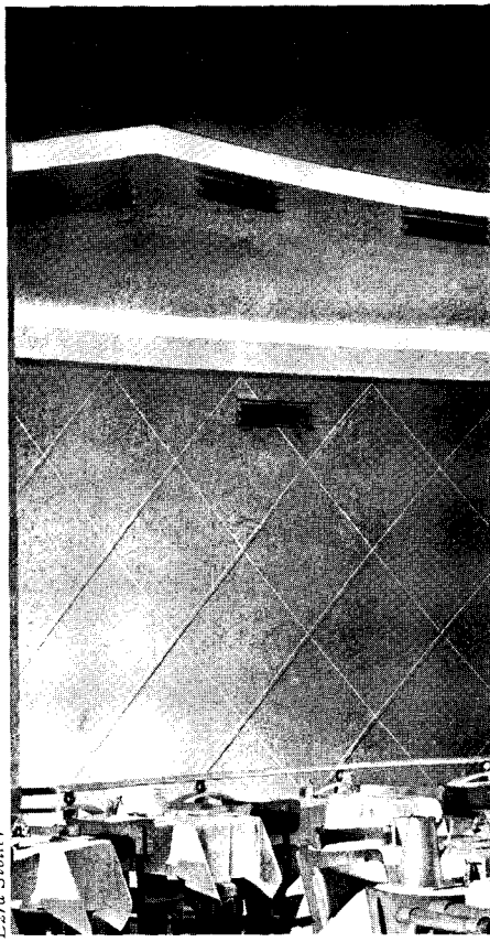
2. Grilles of supply ducts were designed for minimum obstruction to air flow and maximum directional control.
