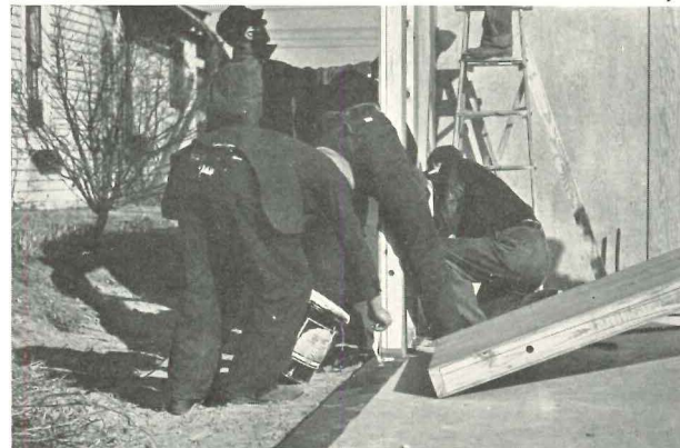
5. Here the white-lead seal is being applied in preparation for the next wall panel. . . .
