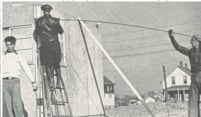
6. Panels are tied together with steel rods and bolted at corners; walls are drawn into rigid units. . . .
