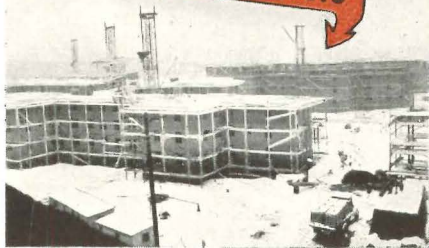
Red Hook Housing Project, Brooklyn, N. Y. General Contractors: Geo. A. Fuller Co., New York City. Mason Contractor: J. H. McNally Const. & Engr. Co., New York City. Associated Architects: Alfred Easton Poor, Supervising Chief, F. T. Fee & W. T. McCarthy, William I. Hohausler, Edward J. Rubin, Jacob Moskowitz, William F. Dominick, E. D. Litchfield.
