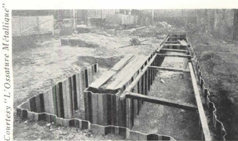
Fig. 6. Many types of corrugated steel piling are used for walls and roofs.
