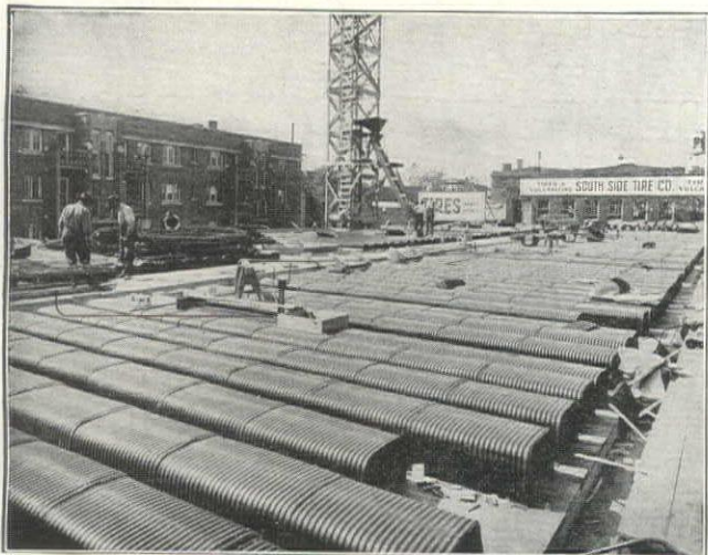
Showing Berger's Pressed Steel Cores installed in the Junius Hotel, Chicago, Ill. Architect, Henry K. Holsman, Chicago. Contractors, C. A. Moses Construction Co., Chicago.
