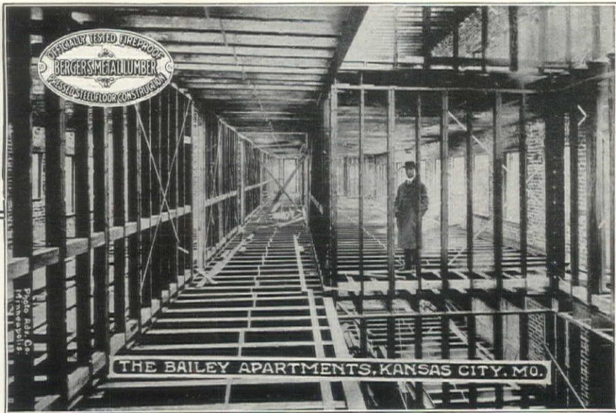
Showing the first, second and third floor joists and partitions. Otis Goddard, Architect.
