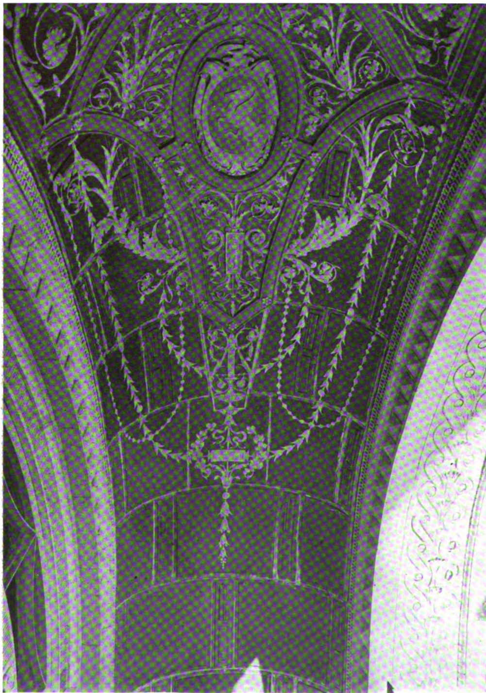
DETAIL OF CEILING IN MAIN ENTRANCE—HADDINGTON BRANCH OF THE FREE LIBRARY OF PHILADELPHIA. ALBERT KELSEY, ARCHITECT.
