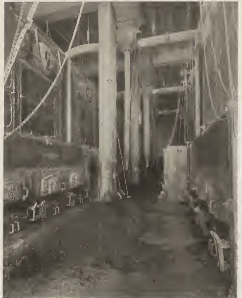
Boiler Room—The Wanamaker Power House. Philadelphia, Pa.
