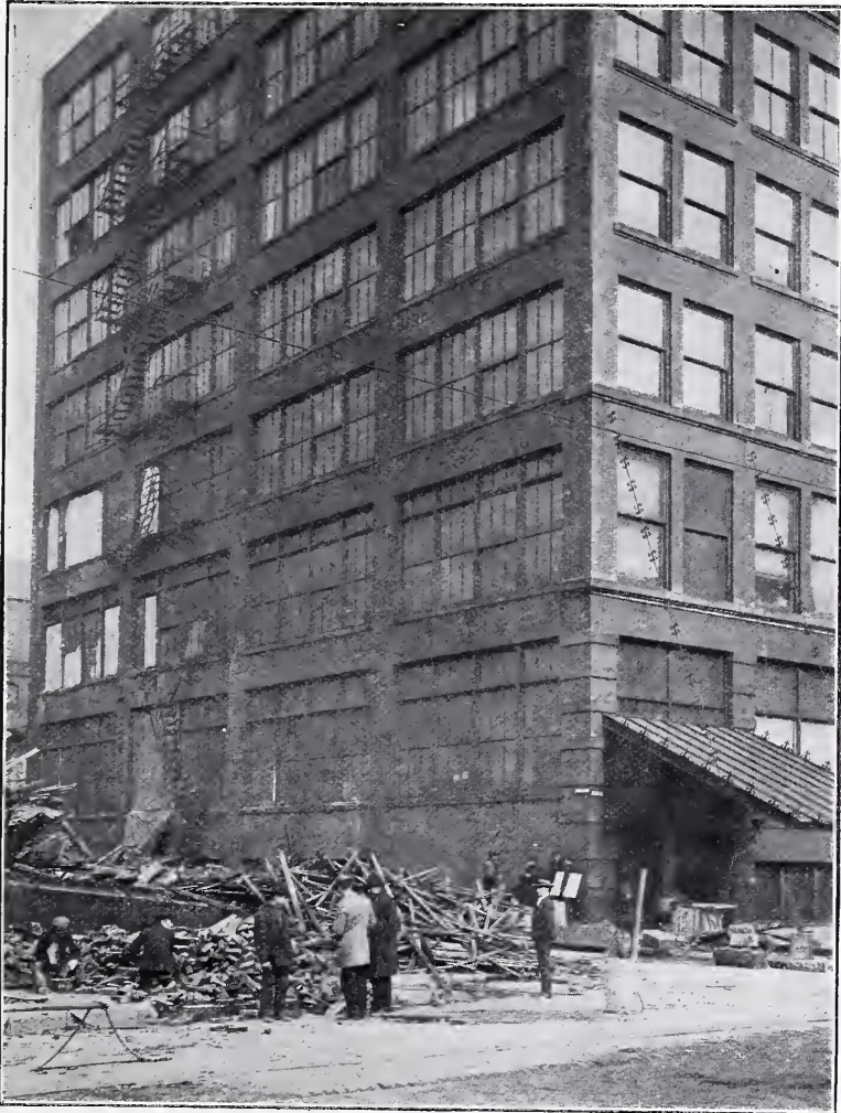
Showing satisfactory fire retardant service of wired glass in metal window frames. Warehouse across 20-ft. alley was totally destroyed. Windows toward rear shown boarded up were broken when side wall of burning building fell.
