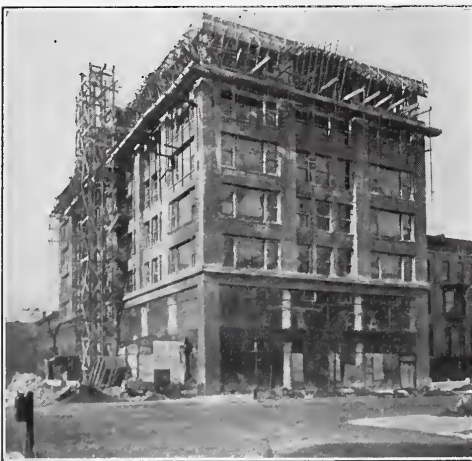
Fig. 8. The Studebaker, Northwest Corner 21st Street. W. E. Walker, Architect. (Showing method of concrete construction.)
