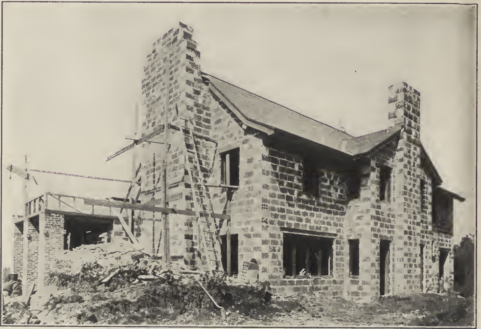
FIG. 5. HOUSE OF MR. MATTHEW SULLIVAN DURING CONSTRUCTION. Canton, Mass. Maginnis, Walsh & Sullivan, Architects.
