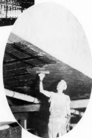
ABOVE: Applying portland asbestos cement plaster finish over wire netting on a duct which is insulated with Corkboard.
