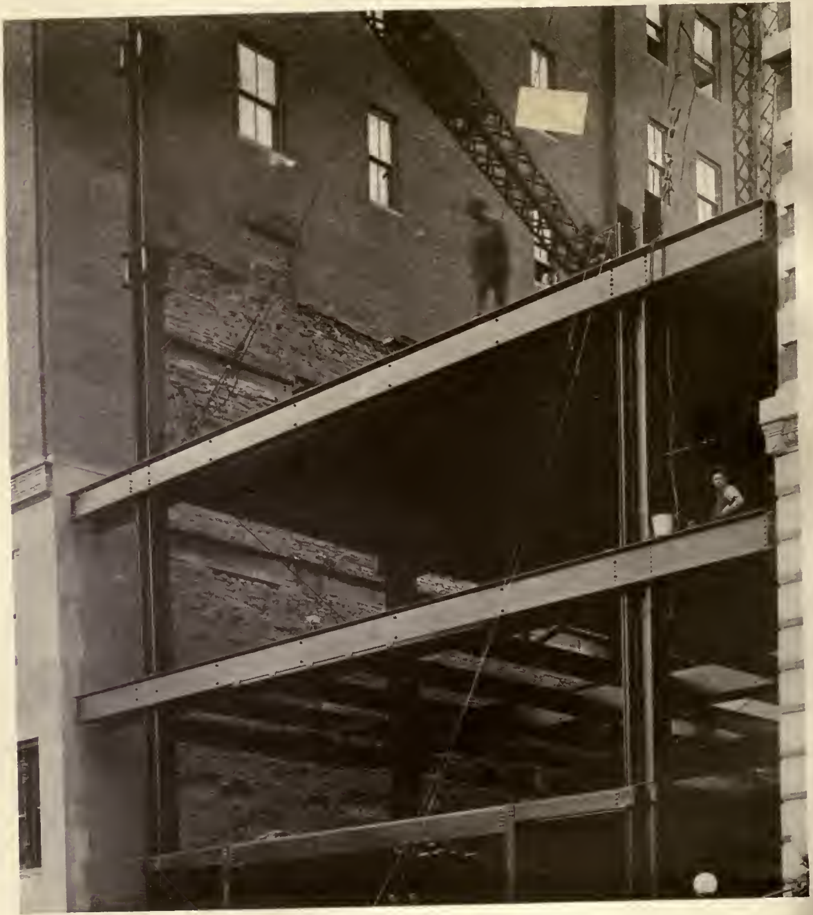
A loft building, 66-70 West 40th Street, New York City, with side walls carried on cantilever ends of floor girders Necarsulmer & Lehlbach, Architects Gunvald Aus Company, Engineers
