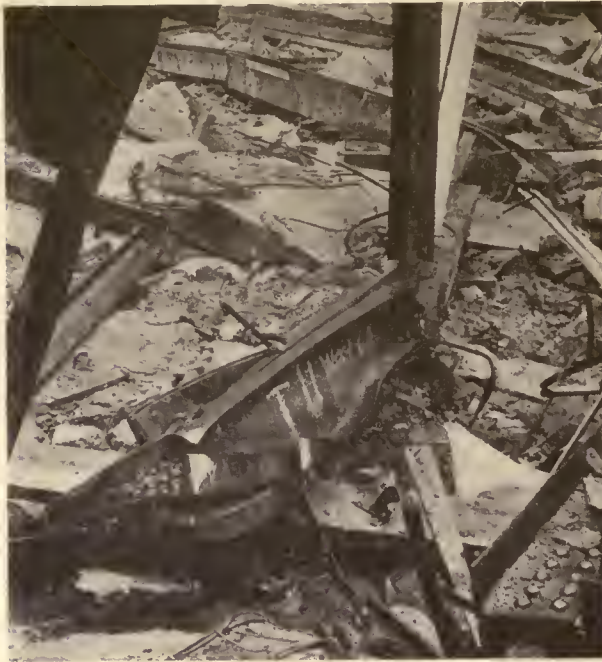
This photograph of the north end section of the bottom chord of truss T-11 shows the effect of a twisting stress, which, combined with the bearing stress, turned the bottom chord off of its bearing on the Columbia Road wall. Note that the west flange at the end is undistorted, while the east flange is curled up against the web. This bottom chord section is the only member found to show evidence of failure before falling. The fact that the corner of the bottom west flange is not injured indicates that a twisting of this member occurred before it struck the floor. Outside of the first panel the truss appears to have been but slightly unlined during the collapse.
