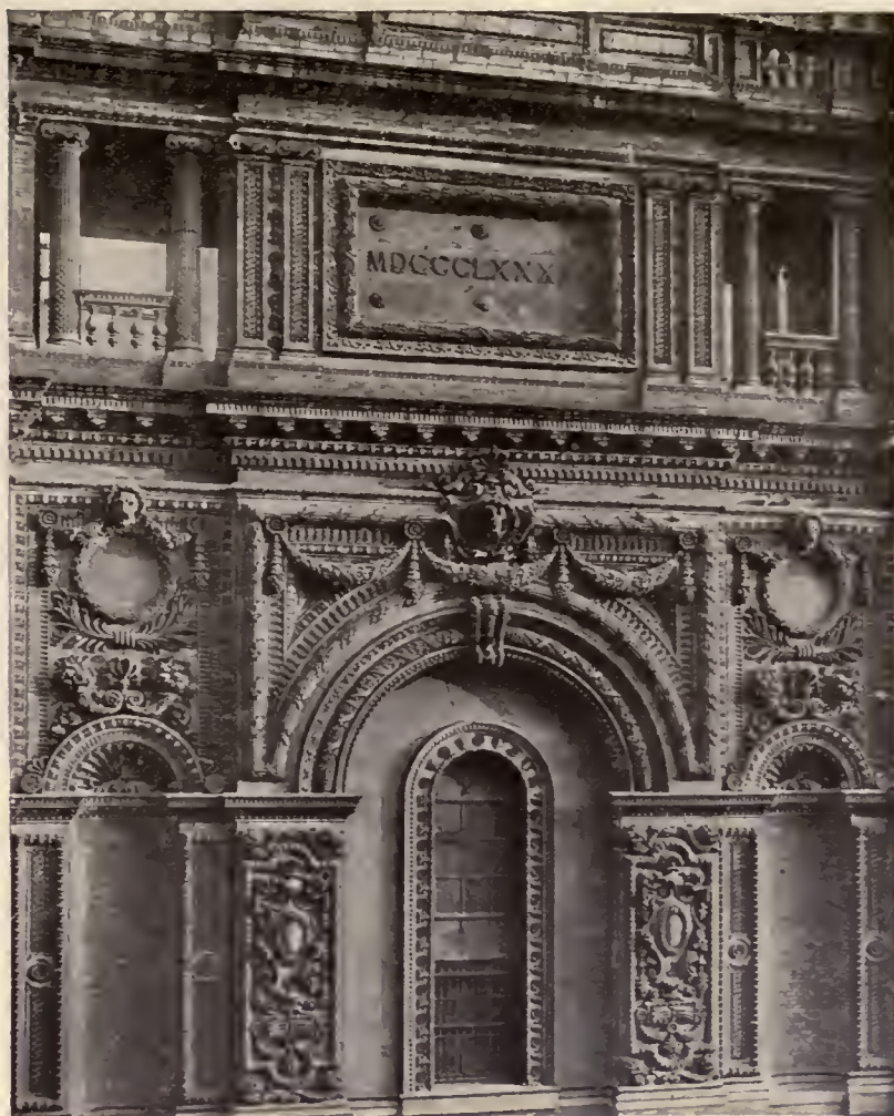
Unretouched photo showing condition of Terra Cotta, March 1st, 1922.
