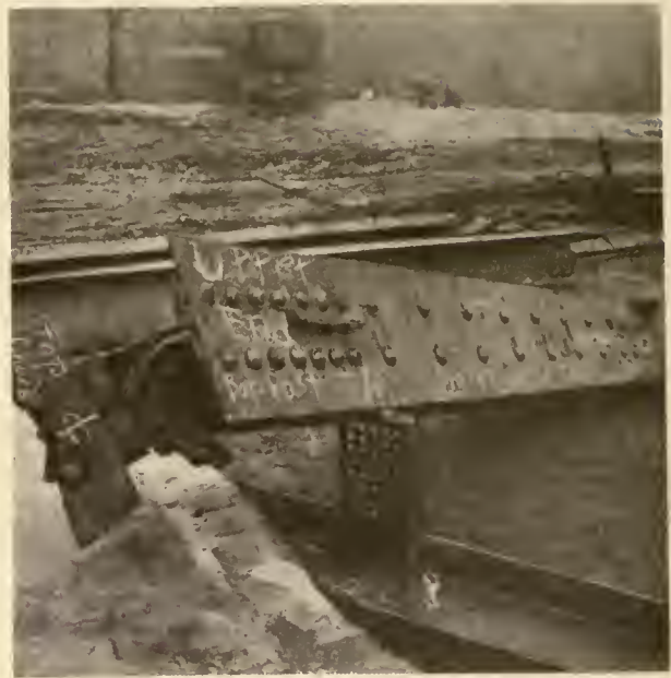
This photograph shows the omission of a cover plate at the upper end of the north batter post of the main truss, and the manner in which the gusset plate buckled toward the west. The stiffness of the heavy upper chord was limited to this half-inch plate. The top chord was cut during the rescue work.
