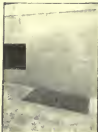
View of Hoistway Sidewalk doors closed flush with pavement, automatically locked.
