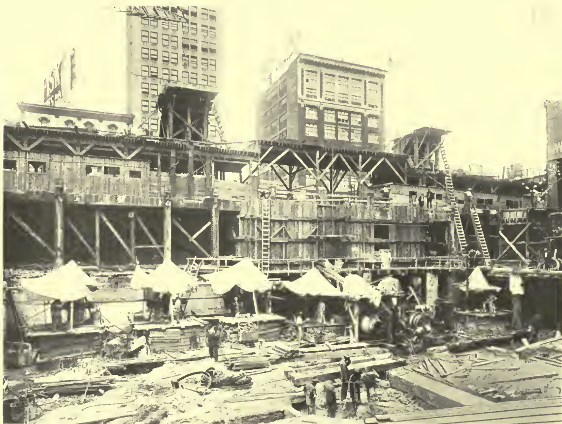
STARTING THE CAISSONS FOR BANK AND OFFICE BUILDING ON THE SITE OF THE OLD HOTEL PONTCHARTRAIN, DETROIT. IN THE FOREGROUND THE CONCRETE MAT IS BEING CUT FOR A CAISSON
