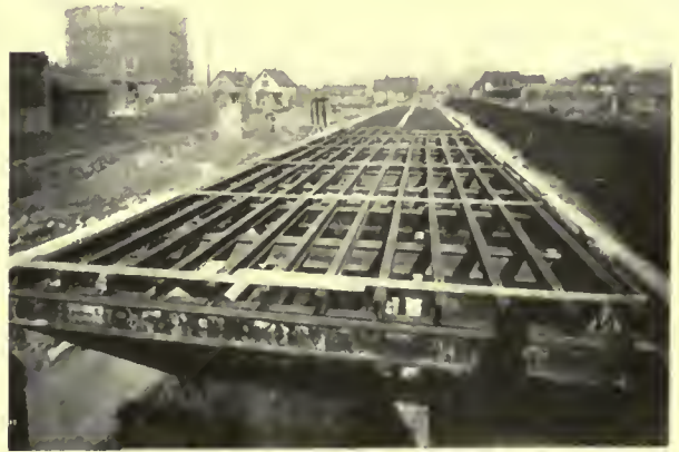
E. J. Woodison Factory, Detroit, Mich. Geo. W. Graves, Architect. Live load 200 lb. per sq. ft. Joists 20 in. on centers. Supported on structural steel
