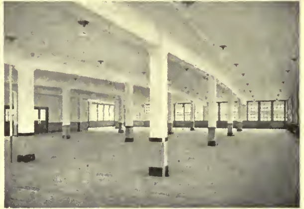
Reinforced concrete. Top floor of an administration building. Long span slabs on beams carried by columns. No intermediate girders. Square columns are inferior to round columns in case of fire.
