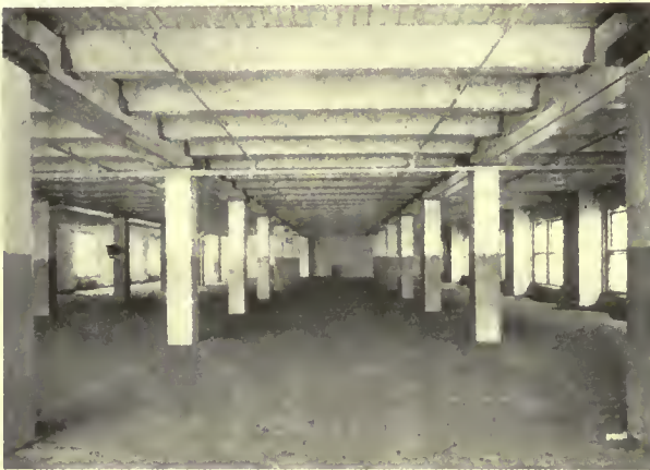
Timber. Semi-mill construction with beams carried on stirrups instead of resting on girders. This effects saving in brick but reduces fire resistance.
