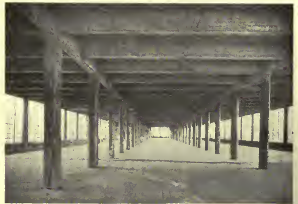
Reinforced concrete. Depth of beams and girders practically equal. Wires go through lower half of beams.
