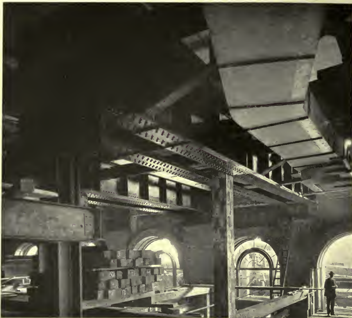
Girders in place under second floor. The ends are supported on steel columns encased in brick piers. The cast-iron column at mid-span was removed after girders were seated and bases were bolted to columns in second story.
