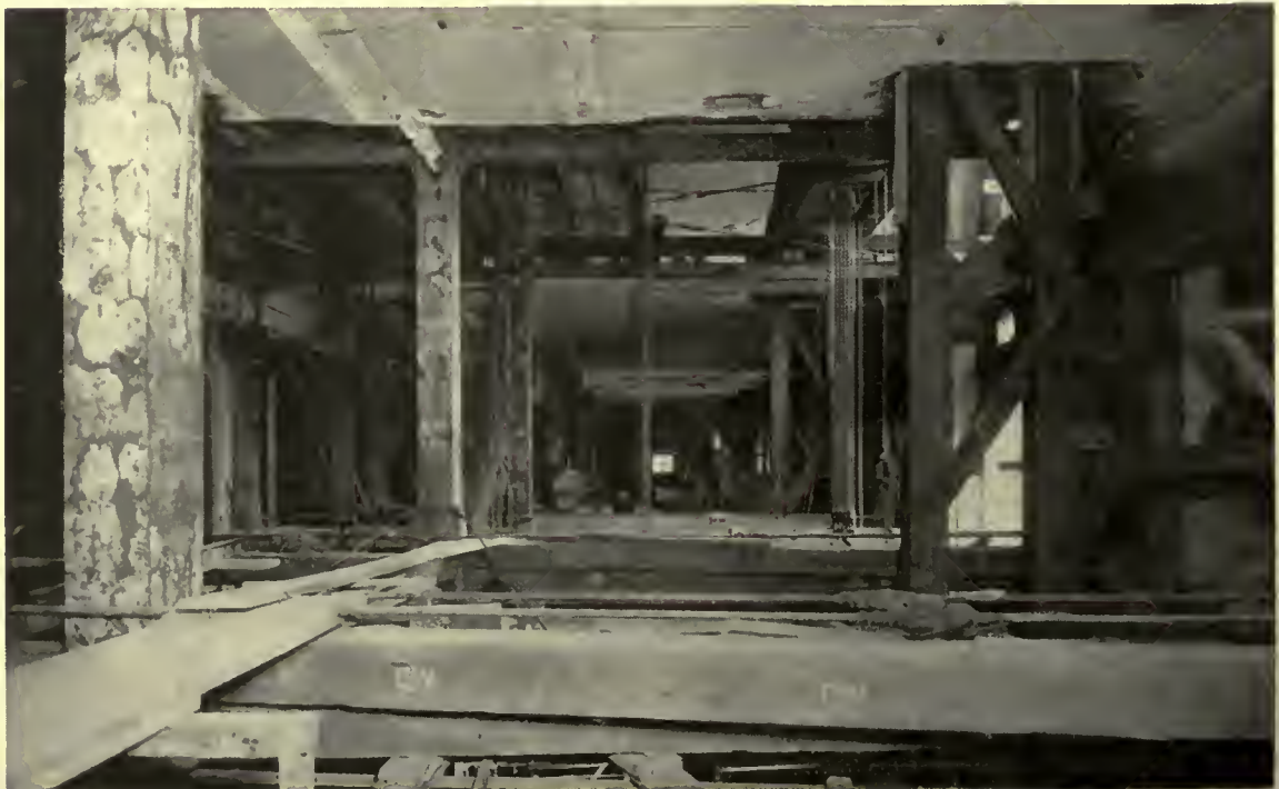
Braced vertical towers supporting heavy trusses on second floor, the lower chords of which are seen at ceiling level with chain blocks in place. Cast iron columns were removed after girders were placed
