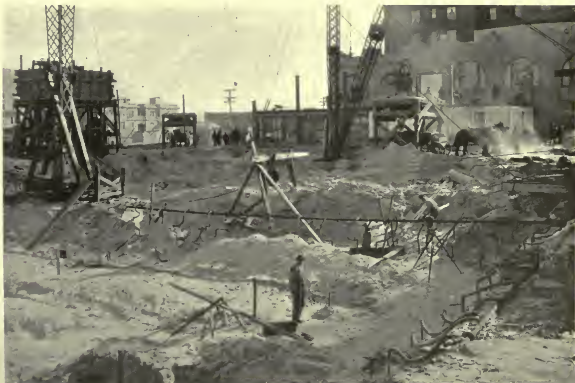
EXCAVATION IN PROGRESS, AMBASSADOR HOTEL ANNEX, ATLANTIC CITY, N. J. This photograph was taken December 15, 1919. The tops of the well points and connecting pipe line used to drain the excavation are plainly visible.
