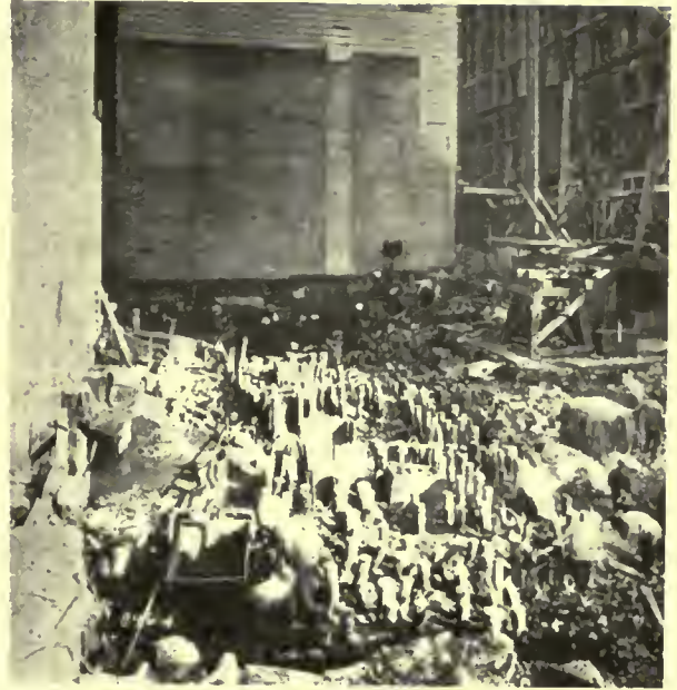
CHURCH EDIFICE ENTIRELY REMOVED Site was excavated to rock and all old piling removed.
