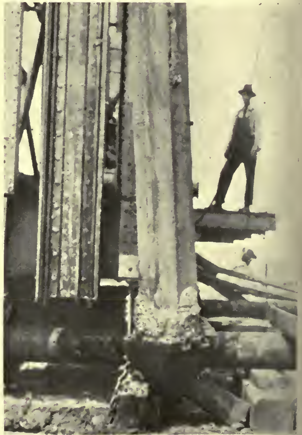
CLOSE UP VIEW, SHOWING CONDITION OF C. I. DRIVING POINT AND CONCRETE
