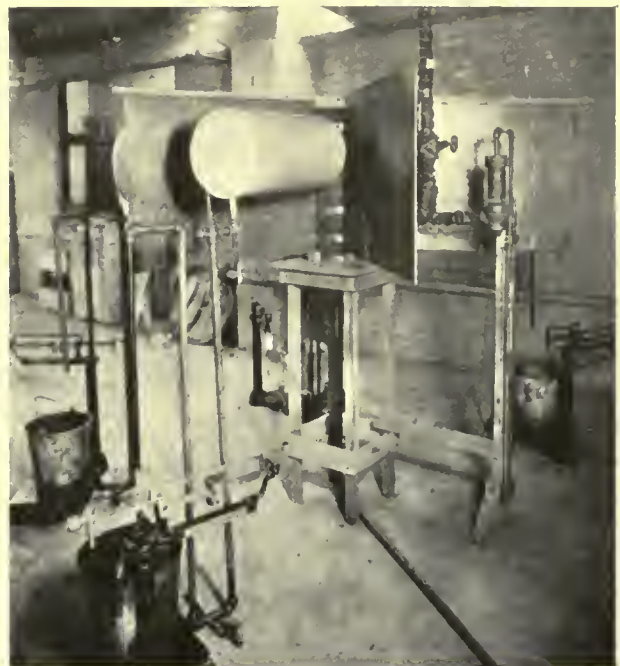
FIG. 2. PHOTOGRAPH SHOWING THE PRINCIPAL OPERATIVE FEATURES OF THE STEAM DRUM PLANT
