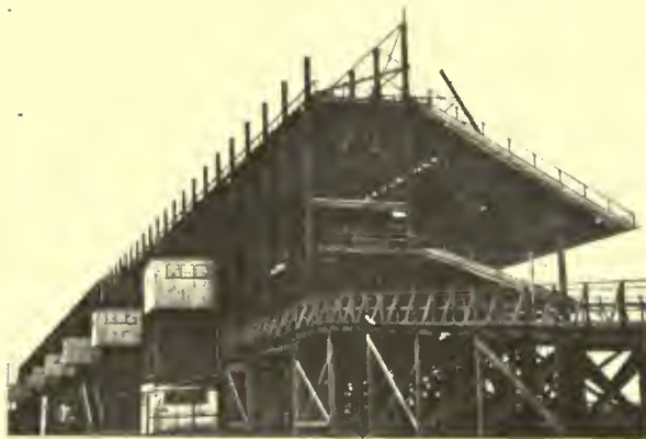
THE GRANDSTAND, WHICH PROVIDED SEATING ACCOMMODATIONS FOR 35,000 PERSONS, IN COURSE OF DEMOLITION
