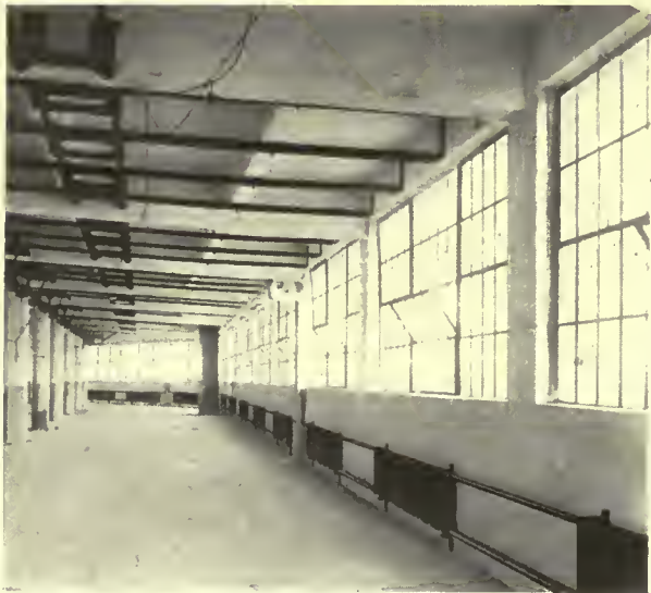
FACTORY BUILDING—THOMAS A. EDISON, INC., ORANGE, N. J. Wall radiators used throughout
