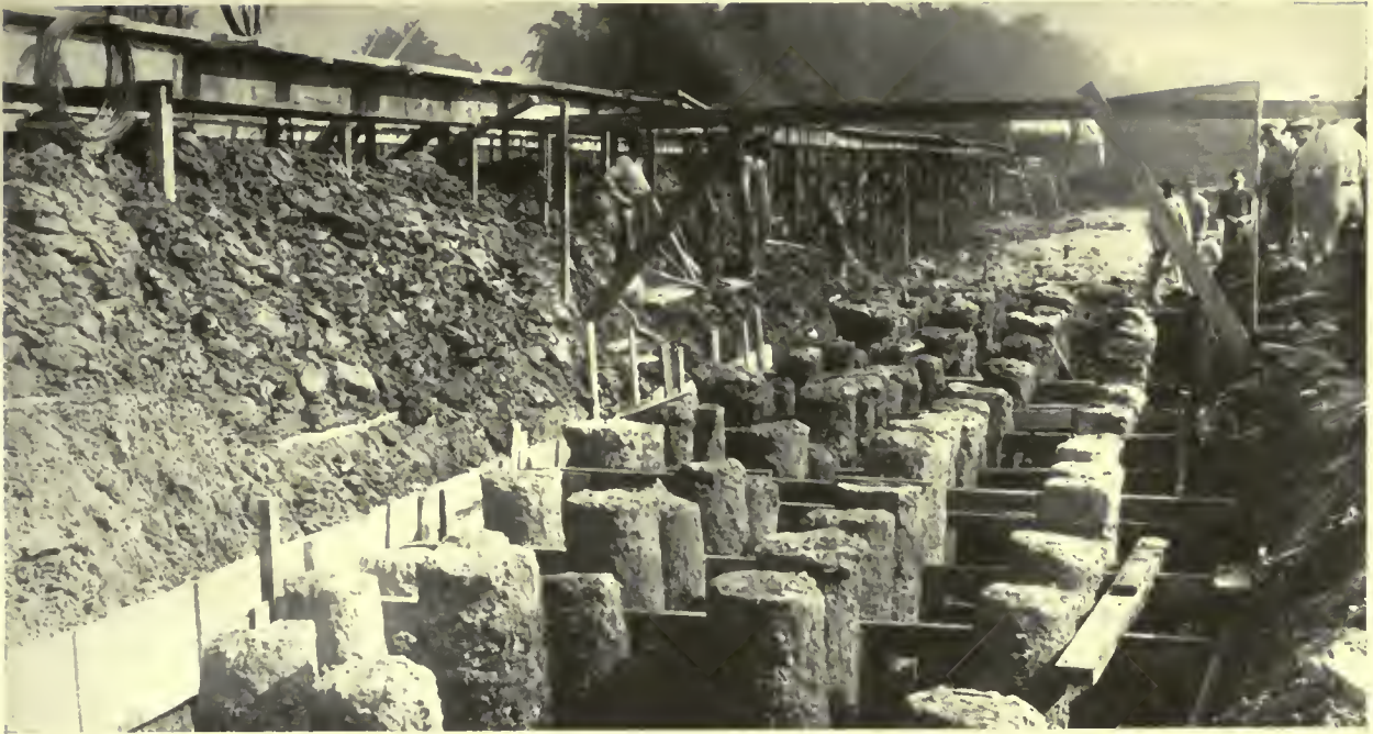
GROUP OF PEDESTAL PILES FOR THE WILLYS-OVERLAND COMPANY'S PLANT AT TOLEDO, OHIO Earth around tops of piles excavated and forms being placed for concrete cap
