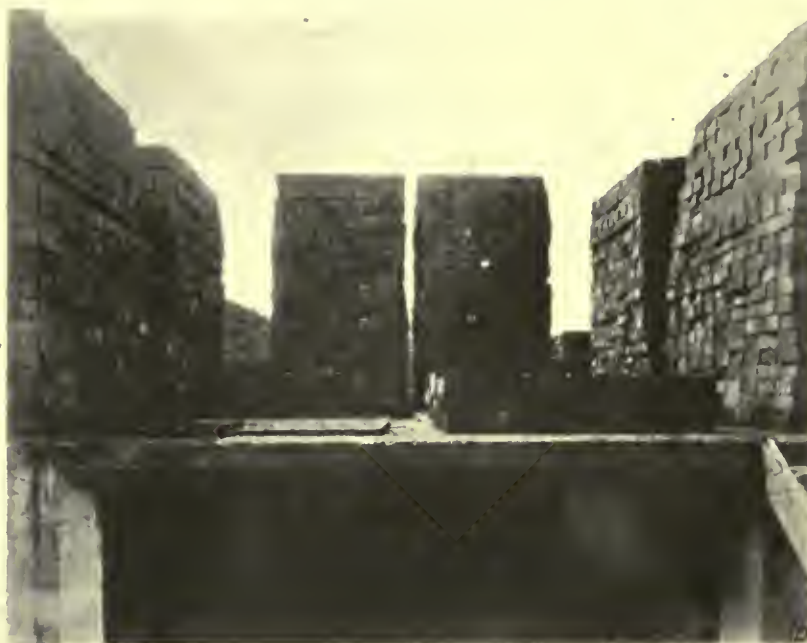
CLOSE-UP VIEW OF SLAB UNDER FINAL LOAD
