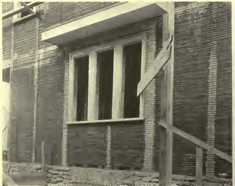
FIG. 4. EXTERIOR VIEW SHOWING PAPER AND REINFORCEMENT IN PLACE. Concrete studs and beams have just been cast.
