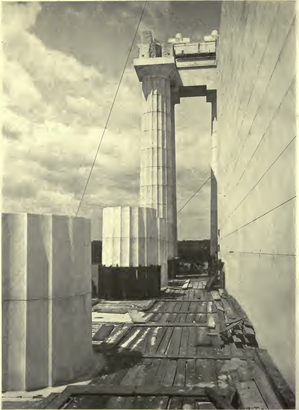
VIEW DURING CONSTRUCTION THE LINCOLN MEMORIAL, WASHINGTON, D. C. HENRY BACON, ARCHITECT
