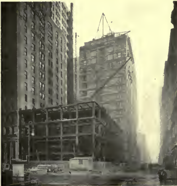
STEEL ERECTION IN PROGRESS Compare adjoining structure at rear with similar view above.
