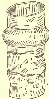
Fig. 20.—Pipe ruptured by Expansion and Contraction of Heat and Cold. (For Scale see Fig. 1.)
