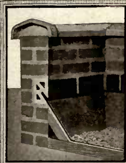
Corner of Roof Showing Brick Wall with Flashing Block and Flashing Installed
