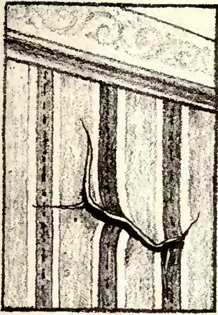
THE DEFECTIVE PLASTER
