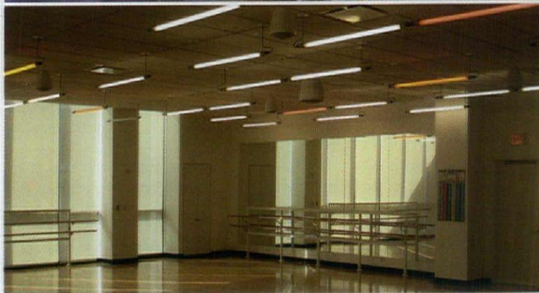
A LED system illuminates the structural glass rear wall of the lobby (top left). The aerobics studio is brought to life by T8 32W fluorescent tubes fitted with colored filters (above). A light pipe was the solution in the swimming pool area providing access for maintenance along the perimeter of the pool deck (top and bottom right).
