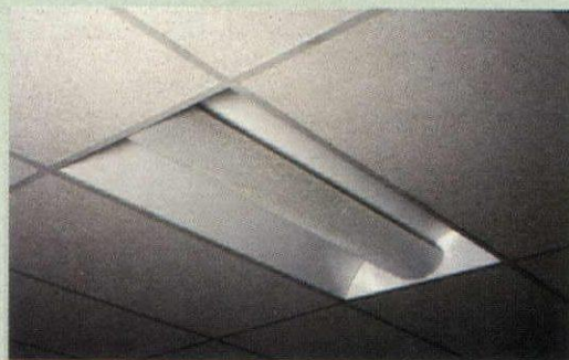
Avante architectural indirect/direct fluorescent lighting
