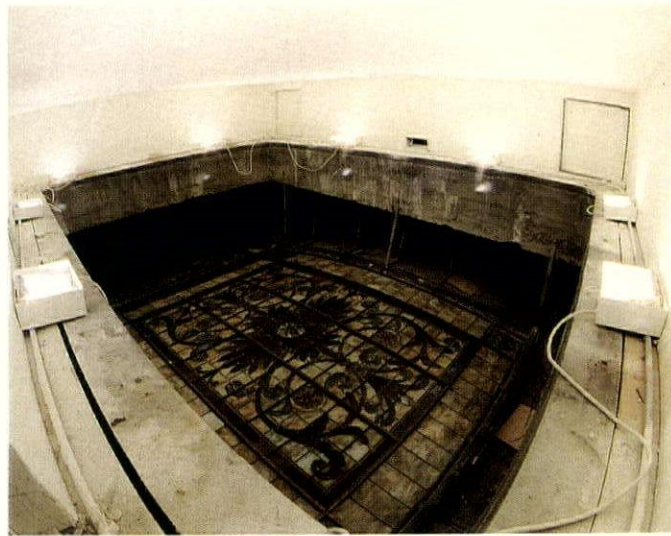
Interior of light box showing indirect 500-watt quartz luminaires.
