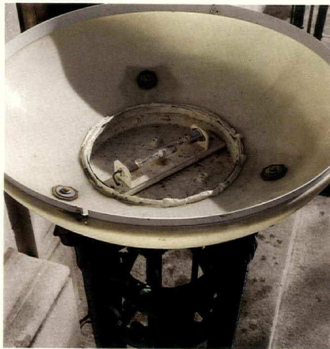
Detail of exterior torchere showing retrofitted metal halide lamp.
