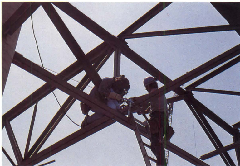
The uniform depth of the steel joists and joist girders added important aesthetic qualities to the arena.
