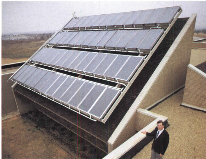
Three state-of-the-art technologies are represented in this installation of equipment atop the Circle T Girl Scout Center in Ft. Worth. The Lennox active solar/variable air volume HVAC system employing advanced electronic controls was simulated by programs developed for Lennox Industries by Control Data's Professional Services.
