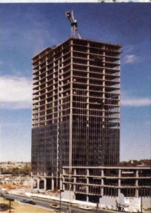
Ceco forming specialists formed a total of 834,000 square feet of flooring and averaged one completed 20,000 square foot floor every six working days.
