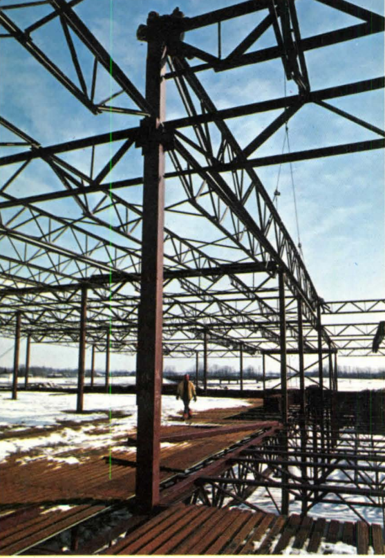
Wide spacing of deep steel joists (6'8" in floors and 7'6" in roofs) resulted in stiffer floor system and saving in the cost of joists.
