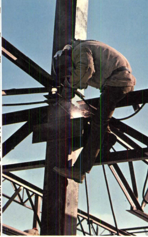
Vulcraft steel joists and joist girders allowed for simple and fast column connections.
