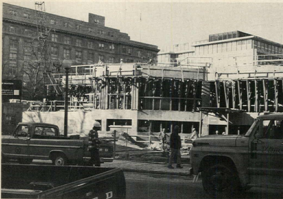
The new headquarters building has the framing up for pouring of concrete on the second floor, and installation of HVAC and security systems has started. The view is from New York Avenue with the Octagon to the left. The seven-story structure will be ready for occupancy in early 1973.
