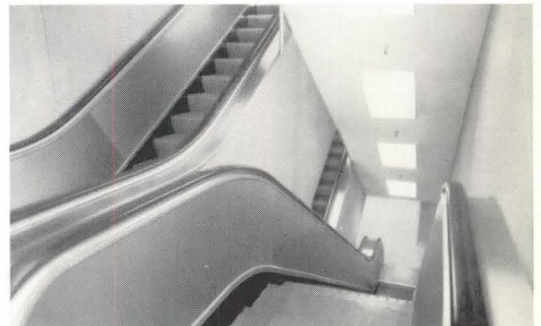
Sixteen Montgomery two-steps-level escalators in the core of the main building.
