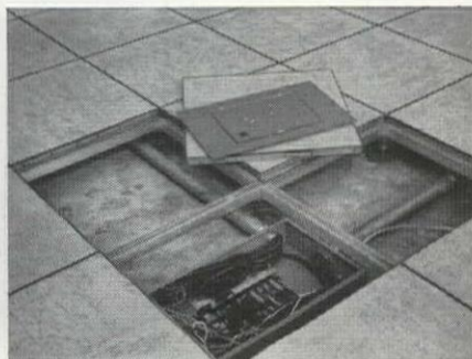
Access to Utilities
