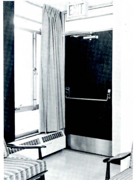
INFIRMARY DOORS where periodically traffic is heavy, are equipped with Norton Series 6100 Uni-Trol, a combination door holder and door closer.
