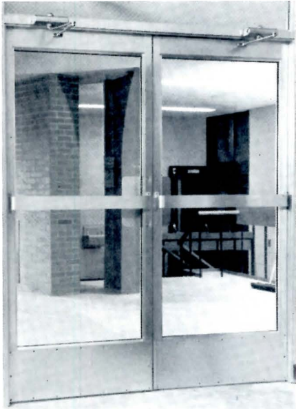
GYMNASIUM ENTRANCE doors with Norton Series 1600 Closers top-jamb mounted. These closers could have been installed just as easily regular arm or parallel arm.
