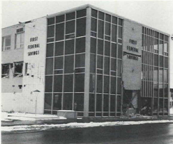
7 First Federal Savings Building: relatively greater damage to unit masonry as compared with curtain wall.
