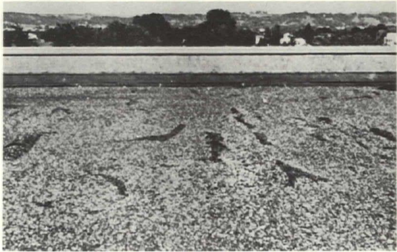
Fig 2—Typical premature failure showing wrinkles, alligator ridges, buckling and blistering of roof membrane as moisture becomes entrapped
