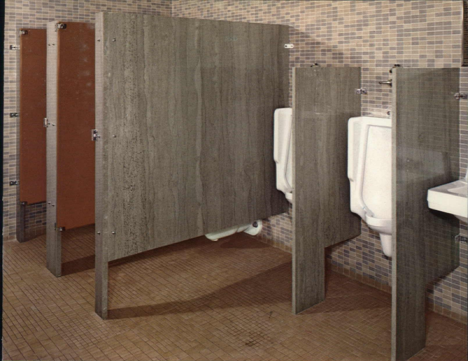
An installation of two Stallpack units with standard urinal screens of matching Ozark Grey Veined marble.
