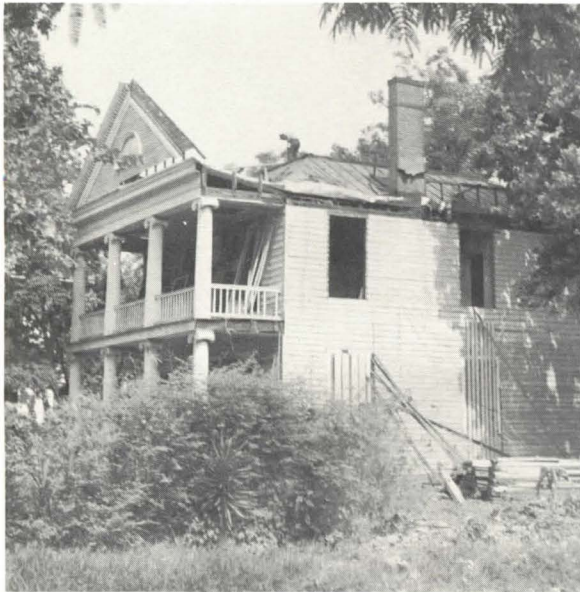
Dismantling uncovered original terne roof and widow's walk, hidden by high gabled roof for many years
