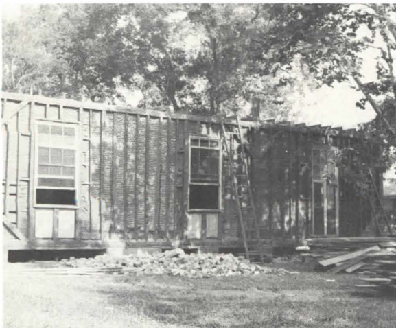
Note hinged panels beneath first-floor windows (covered with siding in 1900), discovered during restoration
