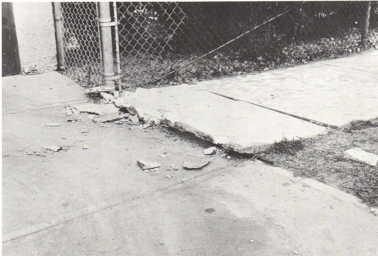
A section of sidewalk slides up over its adjoining walk
