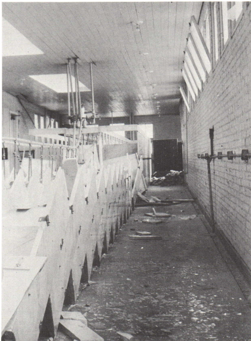
Marble shower stalls went over like dominoes although an adjacent brick wall shows no damage
