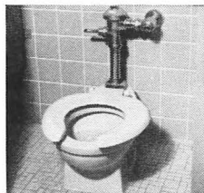
Briggs Tot Water Closets , vitreous china syphon-action models, 10" high, used in the Academy kindergarten.
