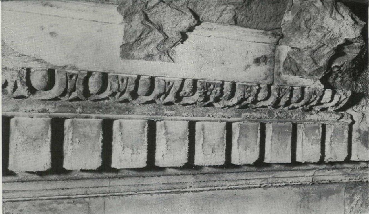
FIG. 8. ORIGINAL MAIN CORNICE AS REBUILT AFTER THE FIRE OF 1814. IN THORNTON'S ORIGINAL DESIGN THIS CORNICE, JUST NORTH OF THE CENTRAL PORTICO, WOULD HAVE REMAINED EXPOSED. LATROBE REDESIGNED THE PORTICO ADDING WINGS AND COVERING THIS CORNICE.
