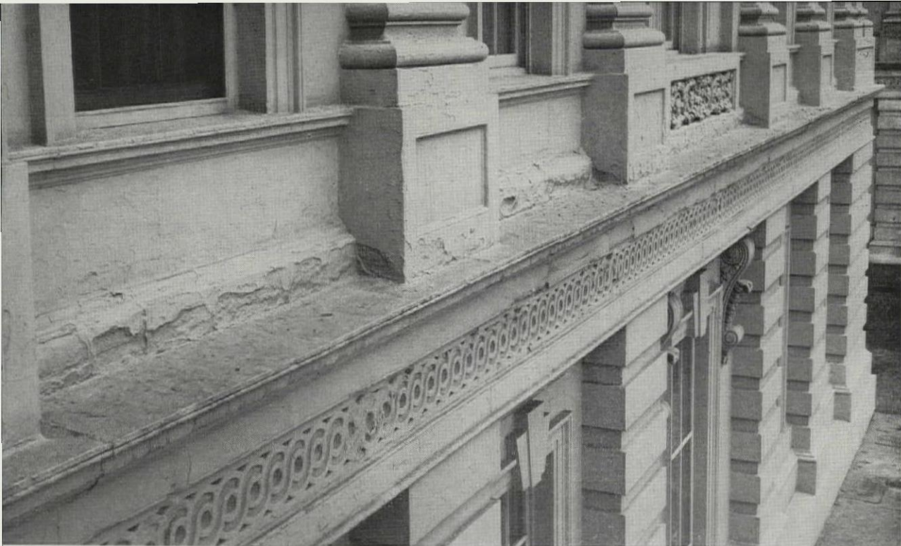
FIG. 9. DETERIORATION OF THE EAST FRONT TAKEN AT THE OLD HOUSE WING OF THE CENTRAL PORTICO AT THE BELT COURSE LEVEL OF THE PRINCIPAL FLOOR.
