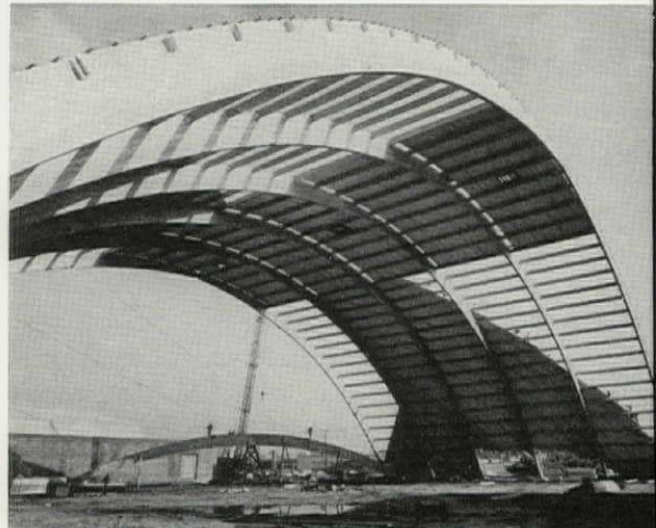
FIG. 10. THIS SHOWS THE 250 FT. SPAN GLUED LAMINATED ARCHES IN ISLAND GARDEN ARENA, WEST HEMPSTEAD, N. Y. THE COST ON THIS JOB WAS APPROXIMATELY $3.00 PER SQUARE FOOT OF FLOOR AREA, INCLUDING THE ARCHES, PURLINS, ROOF DECK, ENDWALL FRAMING AND ENDWALL COVERING.
