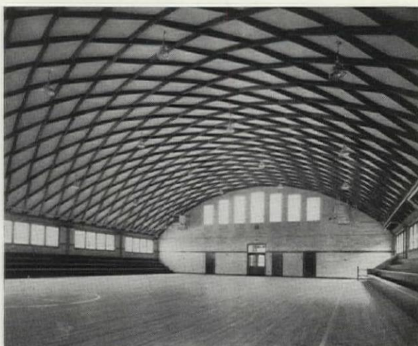
FIG. 3. A GYMNASIUM AT ST. CHARLES, MO., WITH AN 85-FT. CLEAR-SPAN LAMELLA ROOF IS A GOOD EXAMPLE OF LOW-COST ENGINEERED TIMBER CONSTRUCTION.
