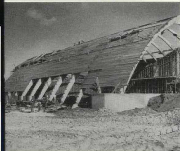
FIG. 8. 4" ROOF DECKING IS COMMONLY USED DIRECTLY ON TOP OF GLUED LAMINATED ARCHES BECAUSE OF ITS DECORATIVE APPEARANCE ON THE UNDERSIDE, ITS STRUCTURAL RIGIDITY, HIGH INSULATING VALUE AND ITS LOW COST. THIS TYPE OF CONSTRUCTION ALSO SAVES LATERAL BRACING.
