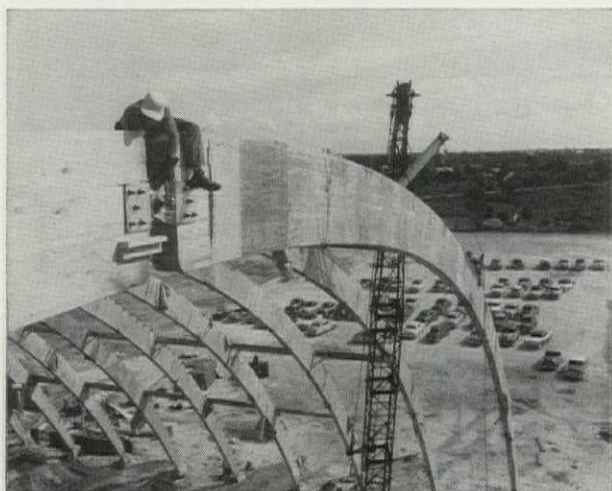
FIG. 4. THESE THREE-HINGED ARCHES SPANNING 248 FT. IN THE JAI ALAI FRONTON AT RIVERIA BEACH, FLA., ILLUSTRATE THE MASSIVE SIZES AND LARGE CLEAR SPANS POSSIBLE WITH ENGINEERED TIMBER CONSTRUCTION.
